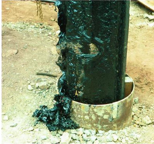
Fig. 7.46 View of a bitumen-coated pile driven through a protective casing The left side of the pile was the pile underside in storage
