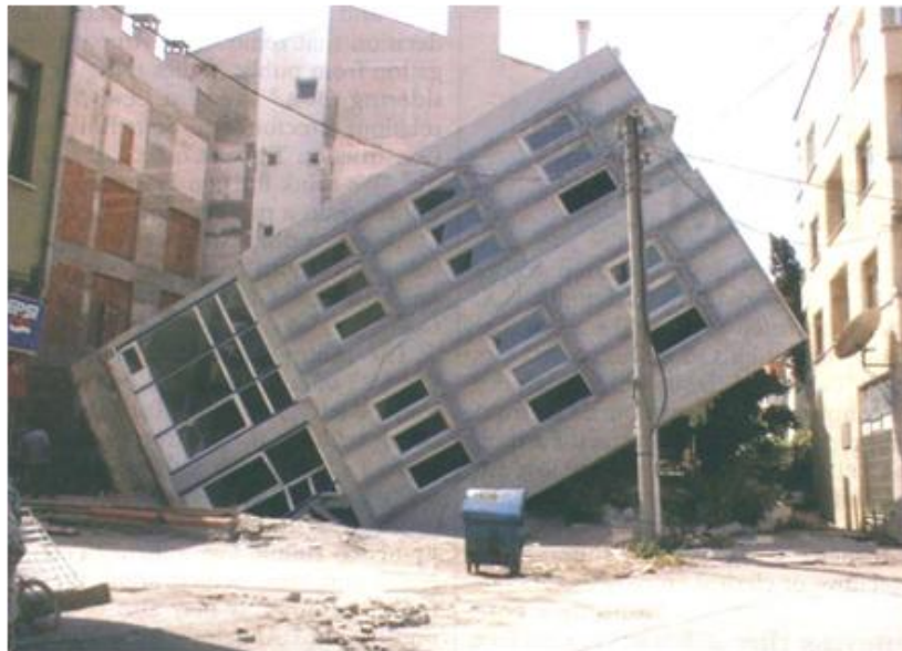
Fig. 2.29 Effect of liquefaction from the 7.4 Magnitude Kocaeli Earthquake of August 17, 1999 in Turkey. Courtesy of Dr. N.J. Gardner, University of Ottawa.
