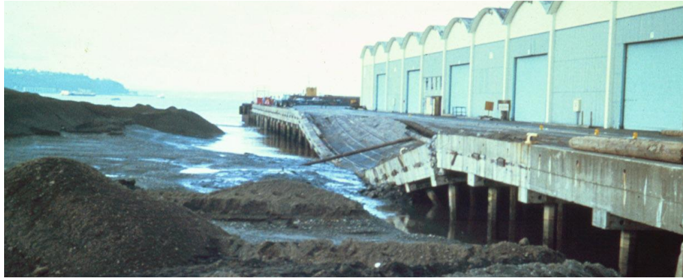
Fig. 7.47 View of the consequence of a hydraulic fill of fine silt flowing against 24-inch piles.
