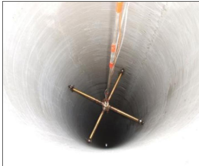
Fig. 8.23 A Glostrex anchor placed down in a cylinder pile (Hanifah and Lee 2006)
