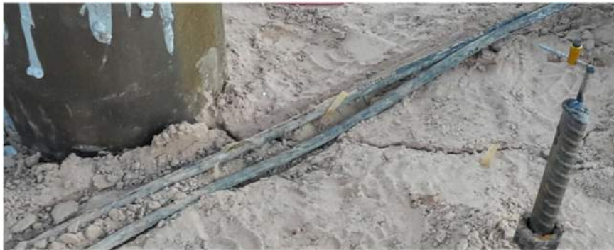
Figure 14. Photographs of cracks in ground surface stretching from one pile toward the next along the side of the group.
