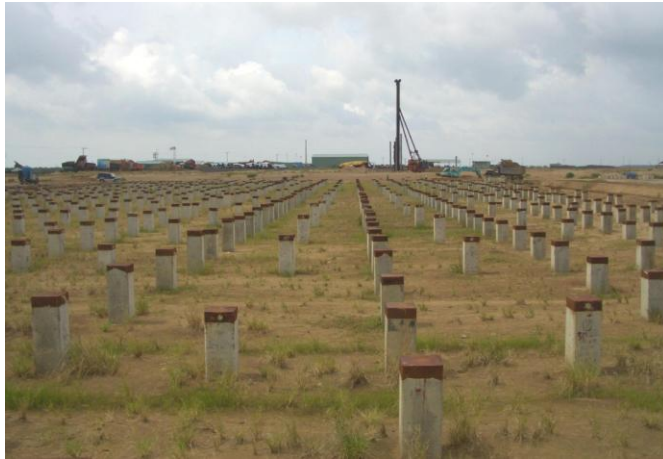
Fig. 14 View on October 4, 2011, from south end of CFS building showing some of the about 750 piles driven for the CFS building. (Authors' photo)
