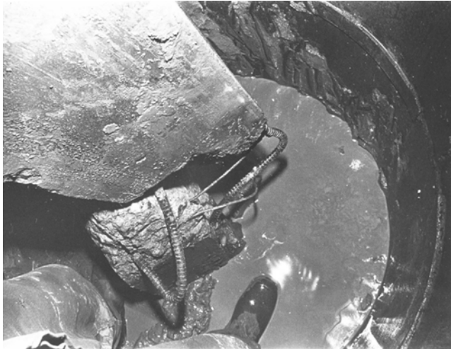
Fig. 5 Detail of the rupture
