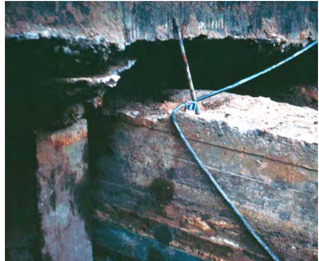
Fig. 3 The settled pile cap and Mega Pile
