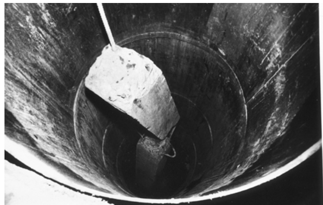
Fig. 4 A ruptured pile excavated in-situ
